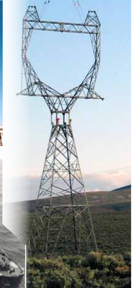
Power transmission line support
