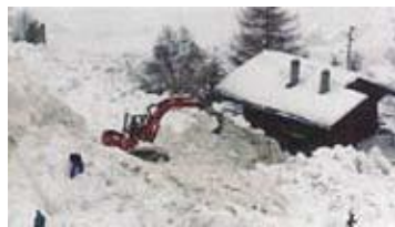
House being cleared from snow
